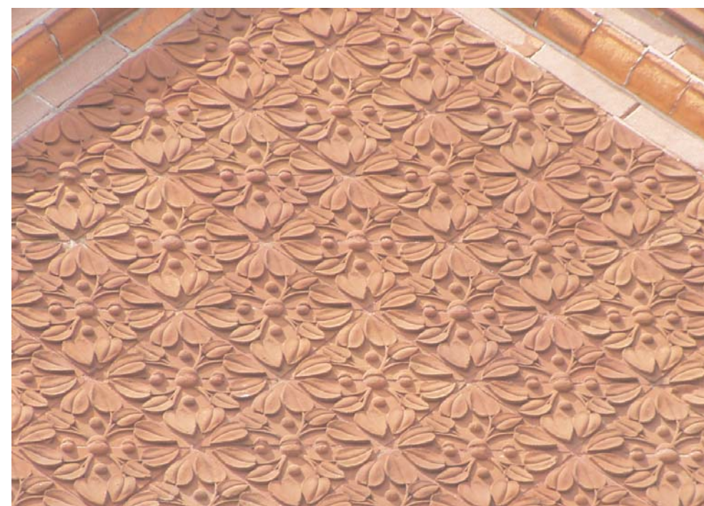
Moulded bricks, tiles and terracotta were popular decorative elements in Victorian architecture.
