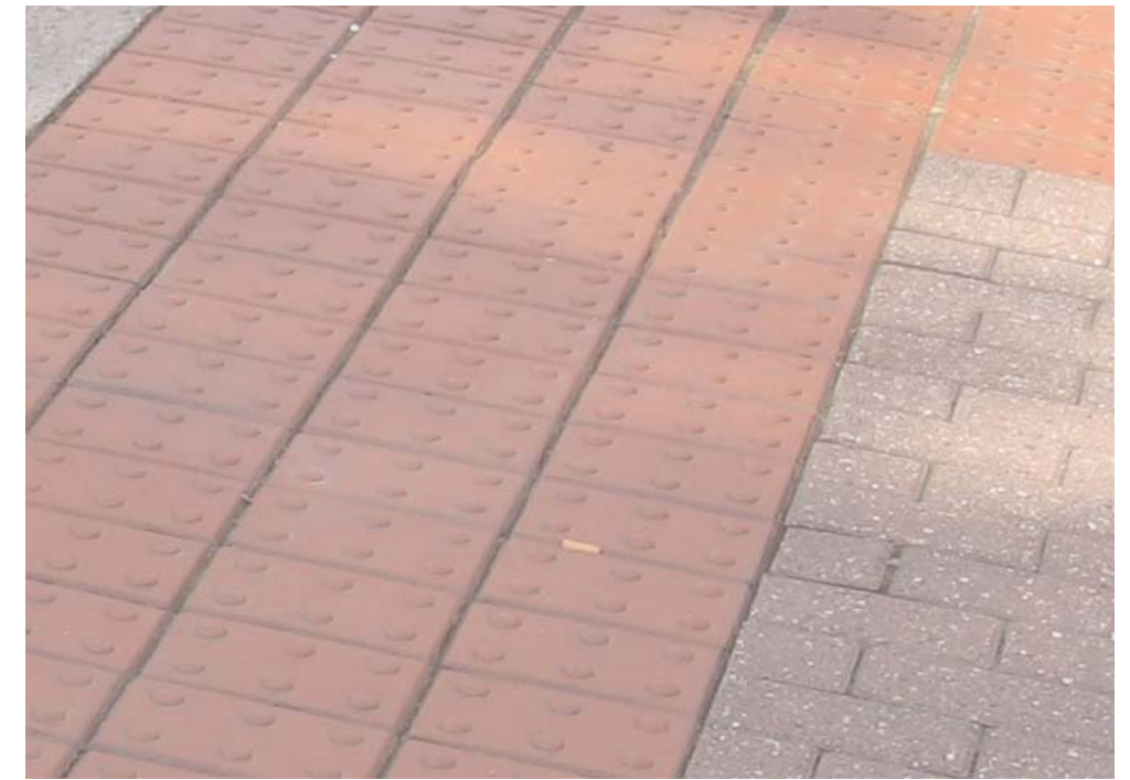
Tactile paving is an important aid to visually impaired pedestrians but needs to be carefully detailed.
