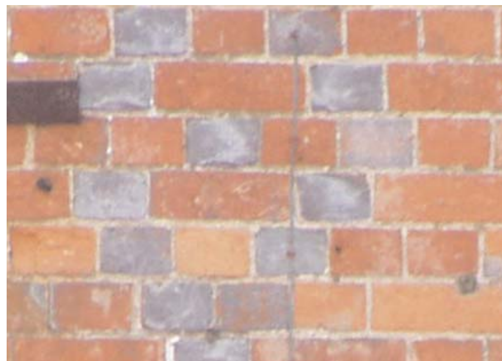
The variety in the red bricks and the use of blue 'headers' creates a satisfying finish.
